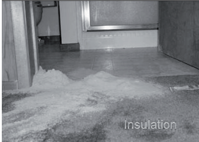
Figure 1. Insulation removed by L. luctuosum in a mountain home in the San Bernardino Mountains, CA.
