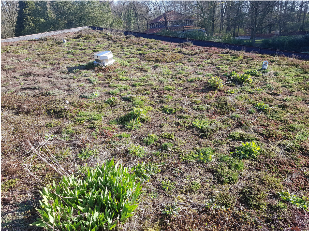
Fig. 3. A photograph of the extensive green roof on top of a pavilion in the Boekenbergpark in Deurne (16.IX.2021). This green roof also had numerous forbs and grasses growing on it in comparison with Roof 1 (photograph: Jeffrey Jacobs).
