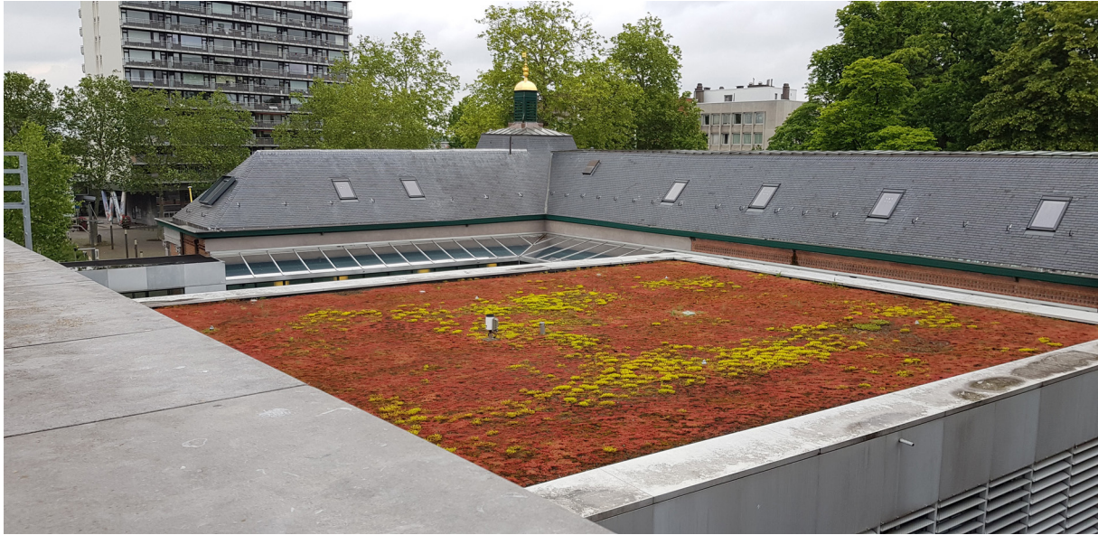
Fig. 2. A photograph of the extensive green roof on the district house in Wilrijk (5.VI.2019). Notice the dominance of Sedum album , which turned red because of the dry weather conditions © Thomas Van Dijck.
